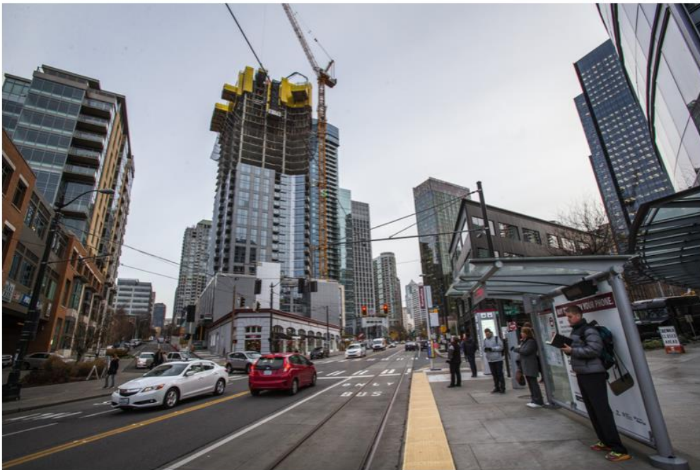
Construction on Stratus overshadows Westlake Avenue. The apartment tower is at 2101 9th Avenue. Photographed Wednesday, December 28, 2016. (Dean Rutz/The Seattle Times)
